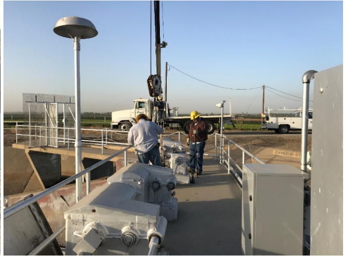
Lindsay maintenance staff continued with the removal of the check gate motors and gearboxes at various locations
