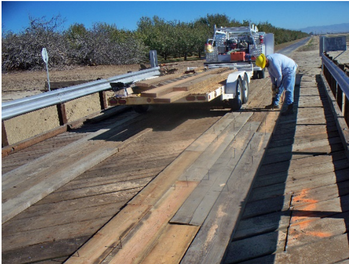
Delano maintenance staff initiated the replacement of broken/wore down bridge timber running pads on eight farm bridges
