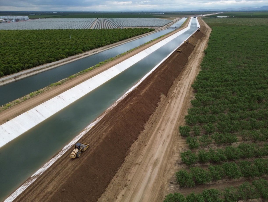
Canal Embankment Placement Above the Canal Lining in Southern Segment of Alignment.
