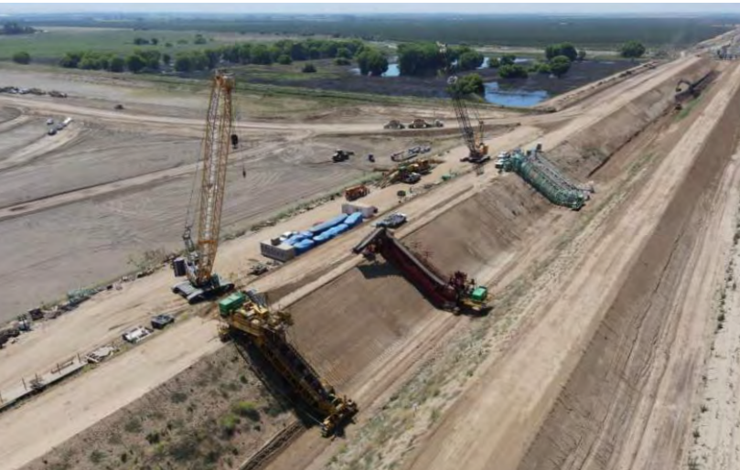
Trimming and concrete lining equipment being setup adjacent to TBID Borrow Site
