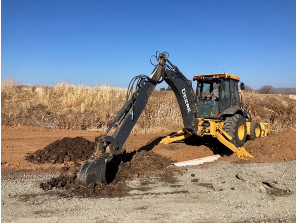
OC staff constructed toe road to eliminate adjacent landowner embankment and bridge traffic.
