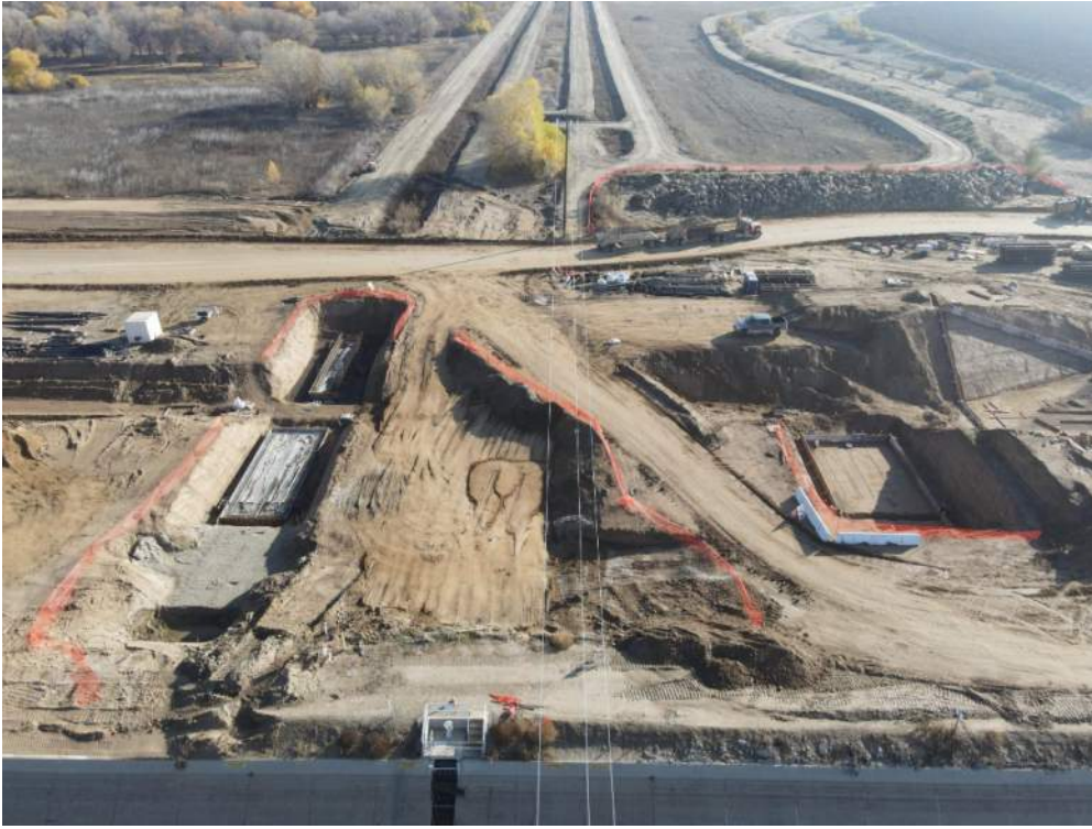
DCTRA Pits and SID S2 Turnouts
