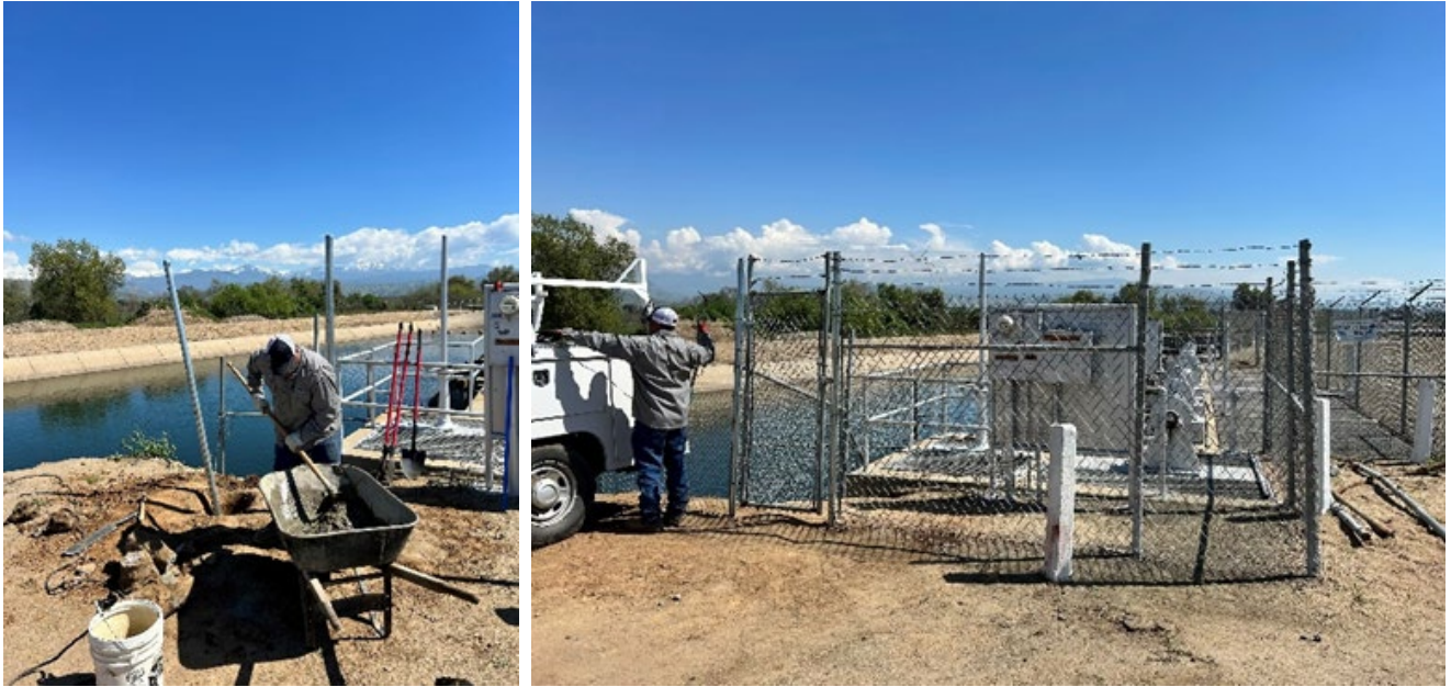
Lindsay maintenance staff inspected fences and made repairs, at St. John's Wastewater.
