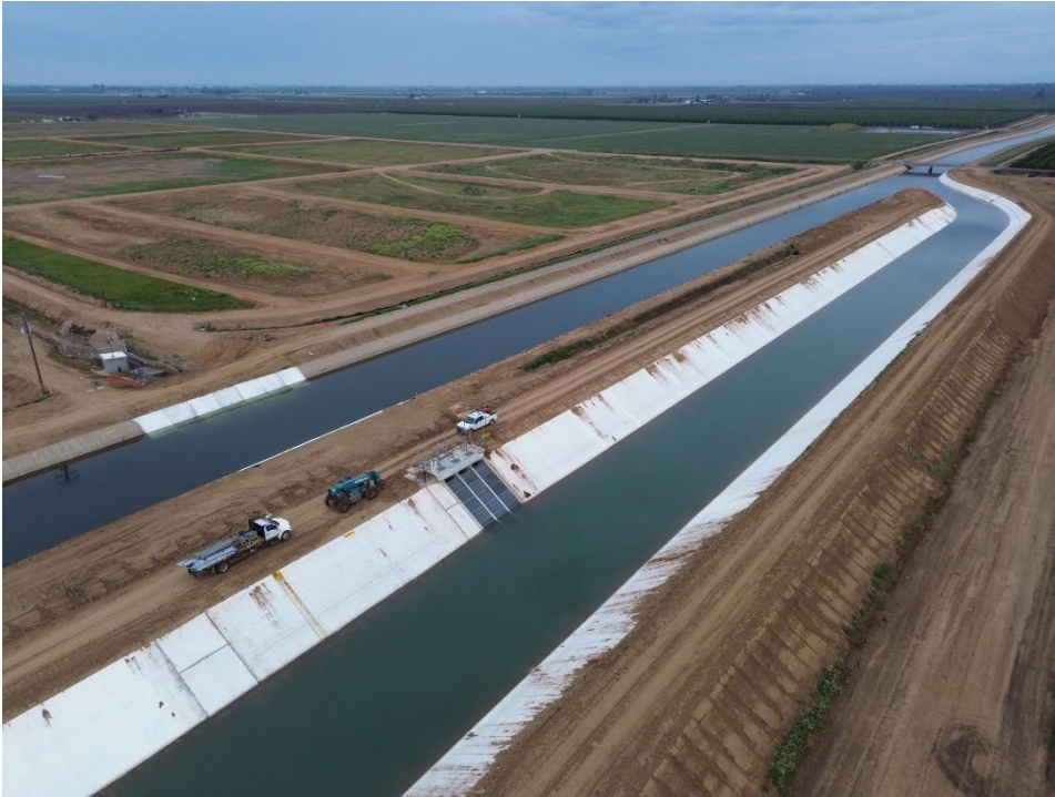
New Parallel Canal at Northern End of Alignment Looking Northwards Towards the North Tie-in.
