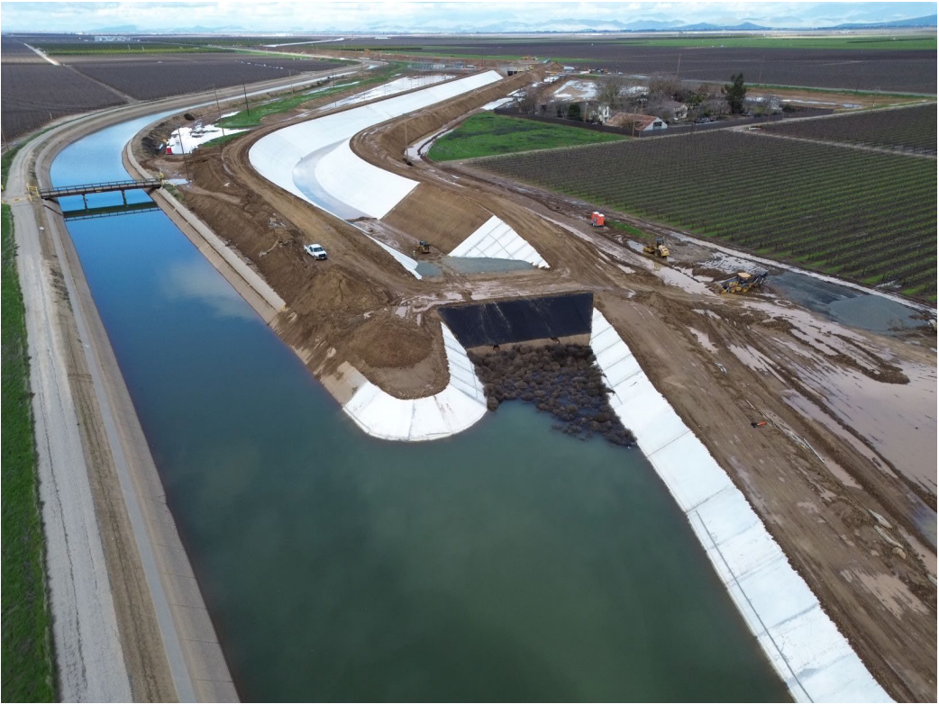
South Tie-in after Completion of Outage Work and Placing the FKC Back in Service
