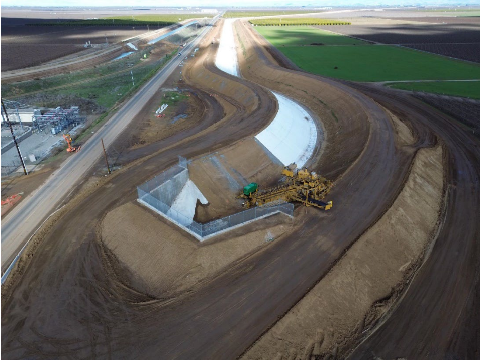
Trimmer Completed Southern End of Alignment on Canal Right and Moved Across Road 192 on Canal Left.
