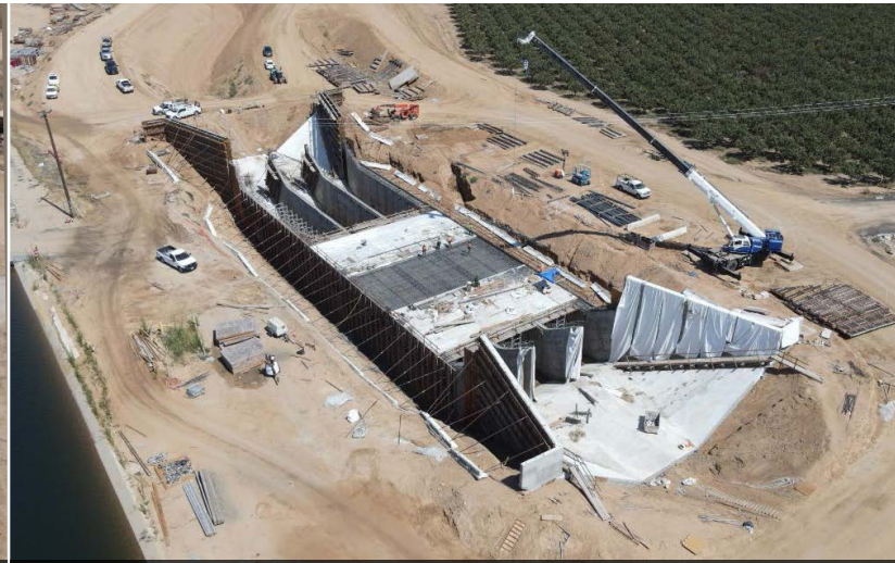
Road 208 siphon transition wall and deck for the flat section in progress
