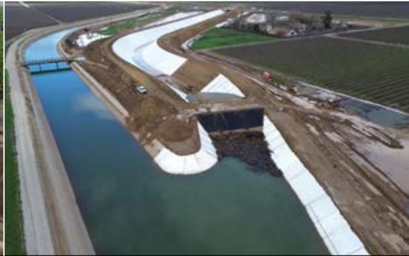
South tie-in after completion of outage work and placing the FKC back in service
