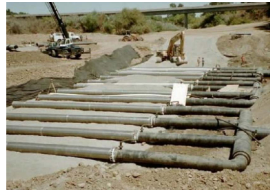
Turlock Irrigation District installed a subsurface diversion system similar to the Environmentally Friendly Water Diversion proposal from the Water Blueprint. Shown above during construction (before being covered by feet of gravel), this system diverts water from beneath the Tuolumne River without harming salmonids in the river.
