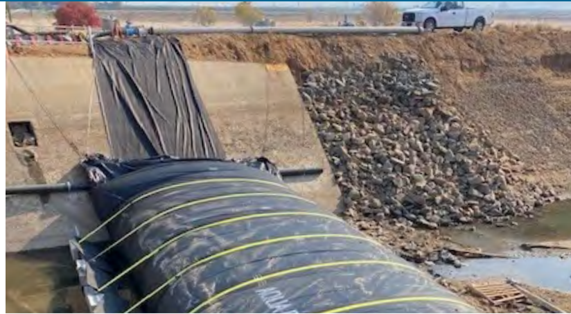
Crews install a temporary coffer dam to store water for use by communities during dewatering.
