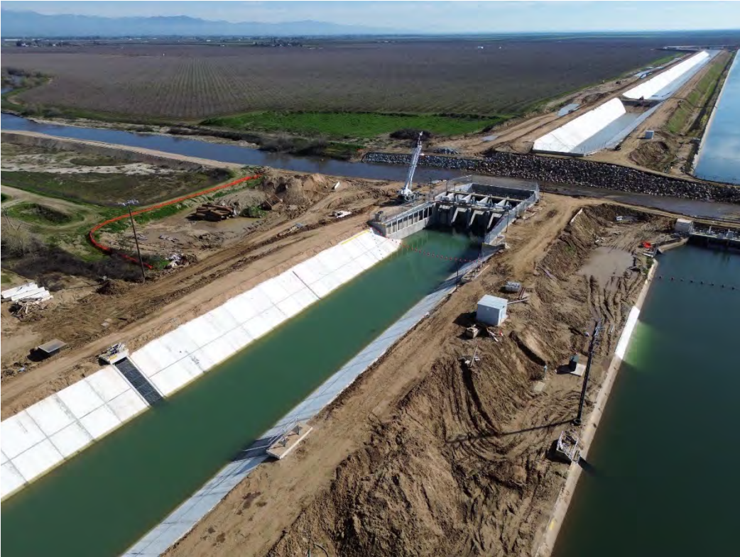
Deer Creek Wasteway and Check Structure and DCTRA and SID-S2 Turnouts.
