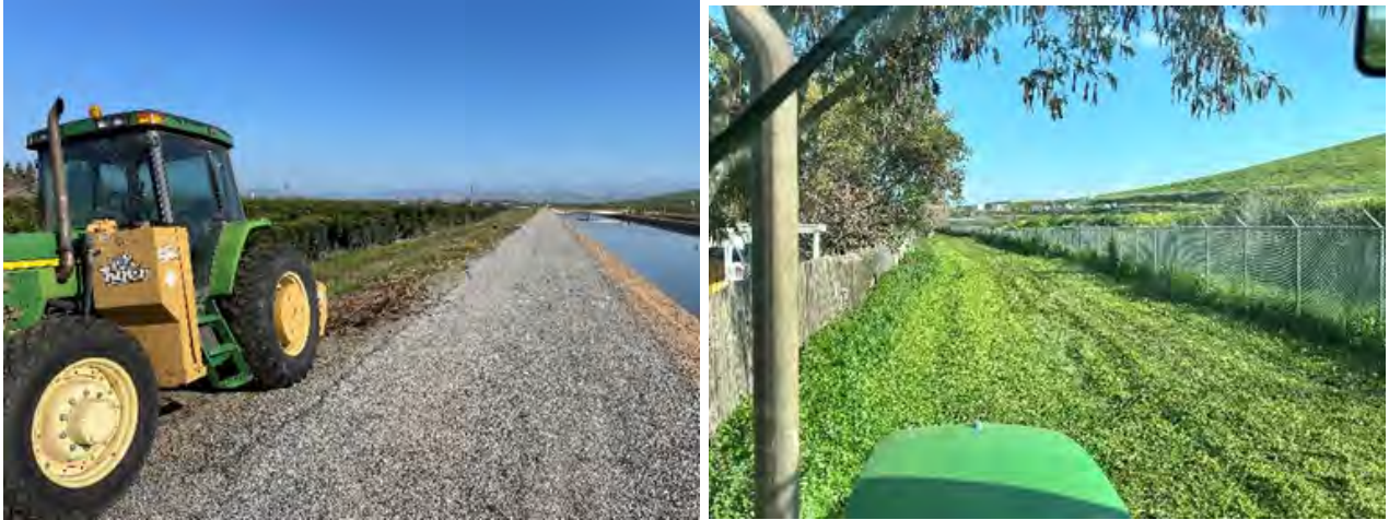
Lindsay maintenance staff clearing tall weeds from ROW and various work sites.
