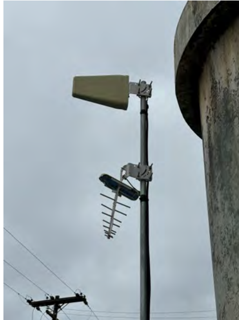
Avenue 56 Vandalized Antenna
