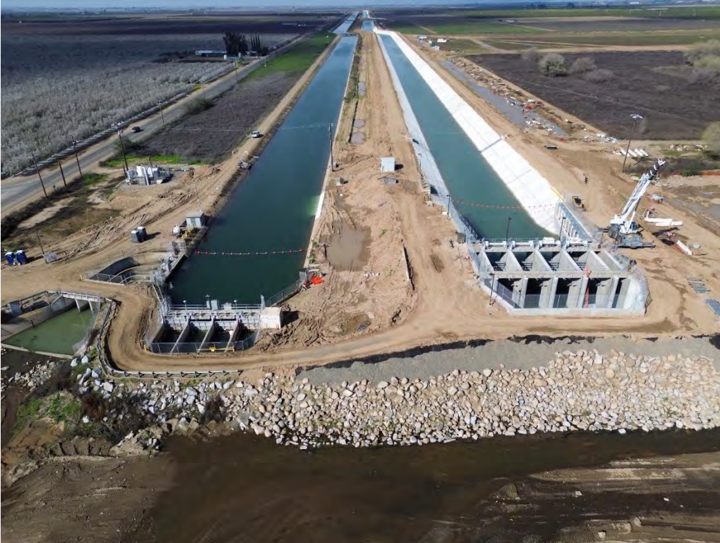
Existing And New Deer Creek Check Structures Looking Northwards.
