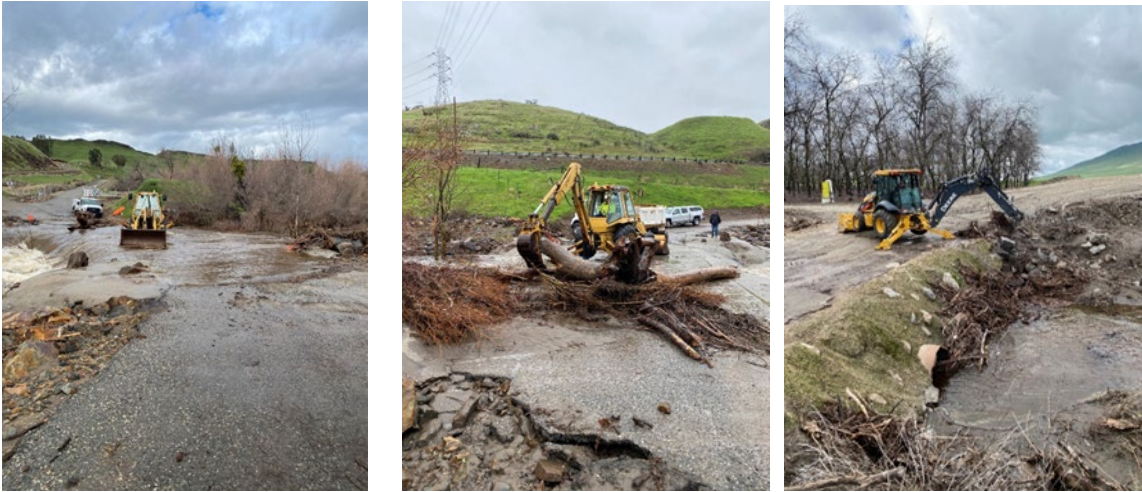
OC staff continued to clean silt and debris out of several cross drainages that were filled after heavy rain.
