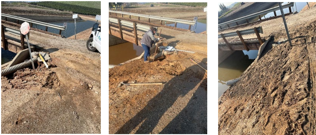
Due to heavy rainfall washouts had to be replaced to avoid additional erosion and potential cavitation behind the liner.
