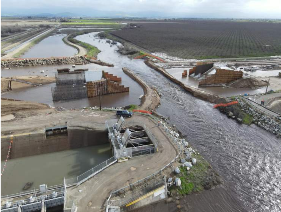
Deer Creek - Temporary berm breach from rain event – 1/10/23
