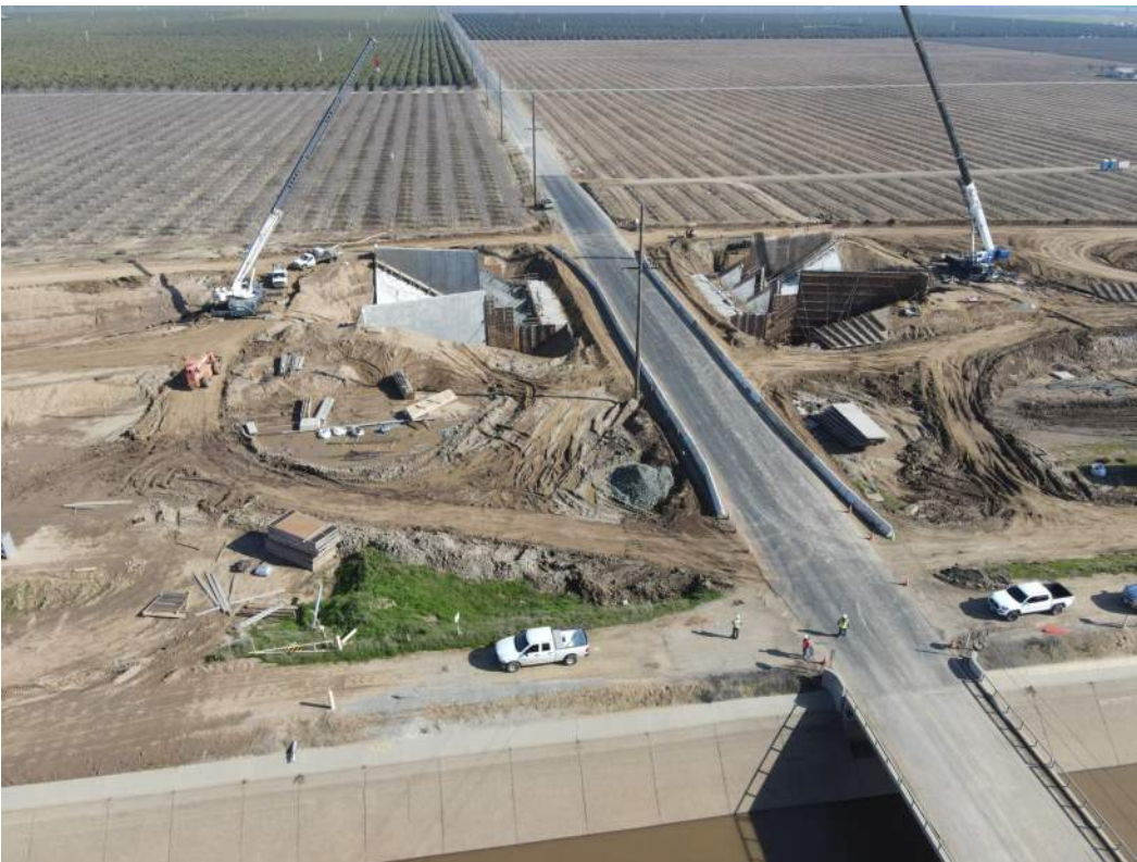
Avenue 112 siphon south transition wall in progress and roadway paved/open to traffic
