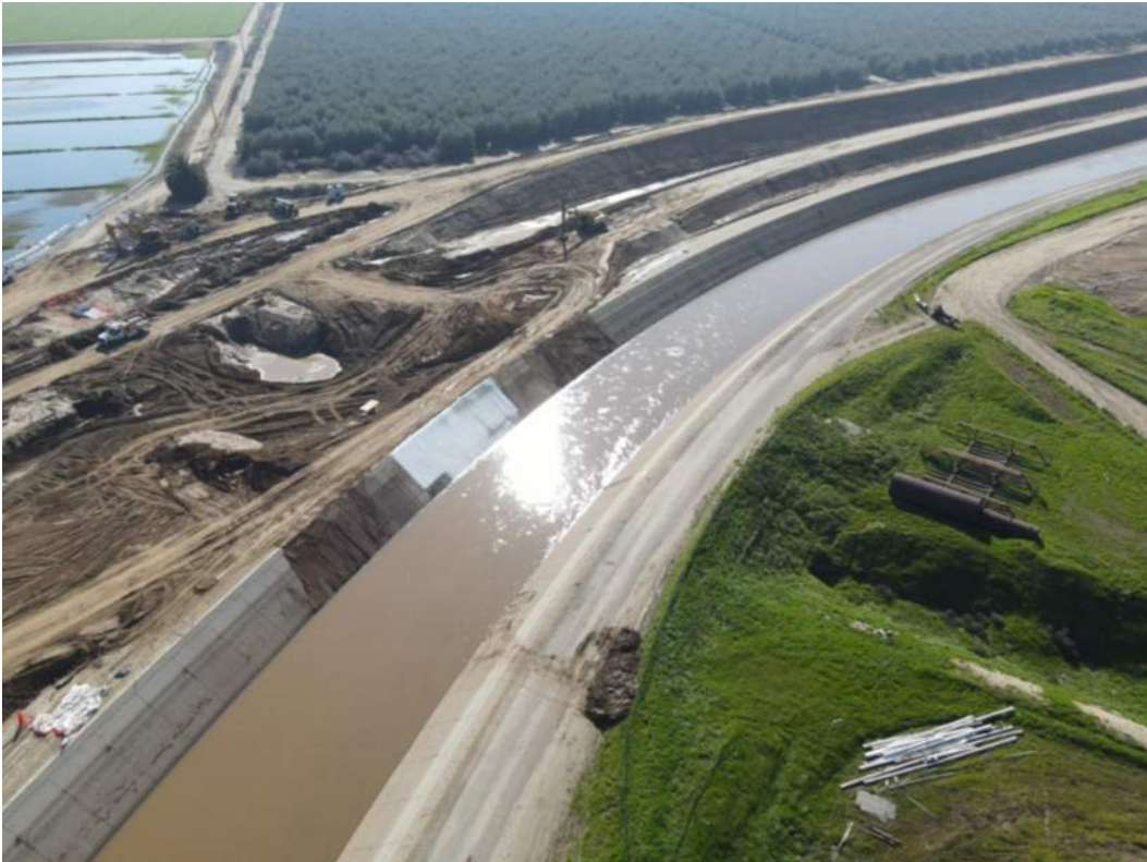
South of Avenue 128 - 5x4 drainage extension box backfilling completed, temporary earthen plug removed and concrete lining replaced- 01/13/23
