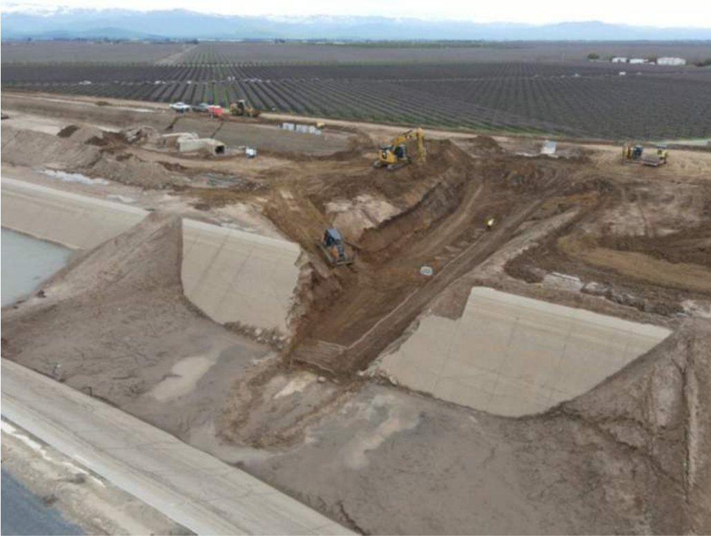
South of Terra Bella Avenue - 5x4 drainage extension box backfilling in progress
