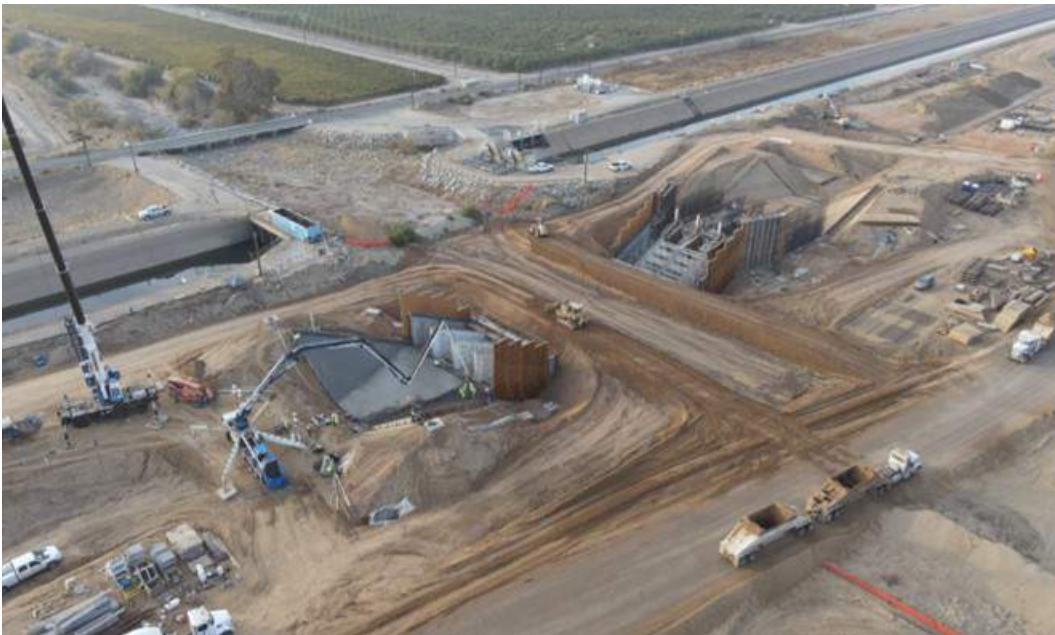
Deer Creek Siphon - Deck Backfilled and Temporary Creek Bypass Berms Being Placed
