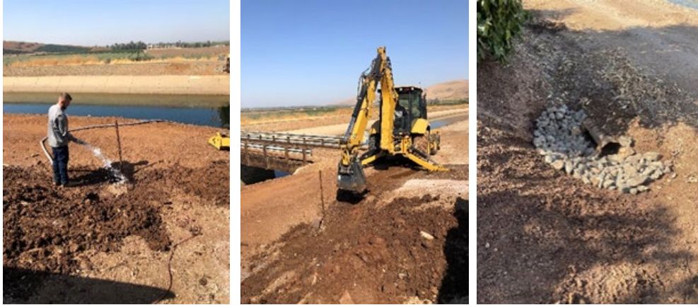
Lindsay staff flushed inlets to remove debris in preparation of winter rains, and created a clear drain and placed a riprap to reduce buildup
