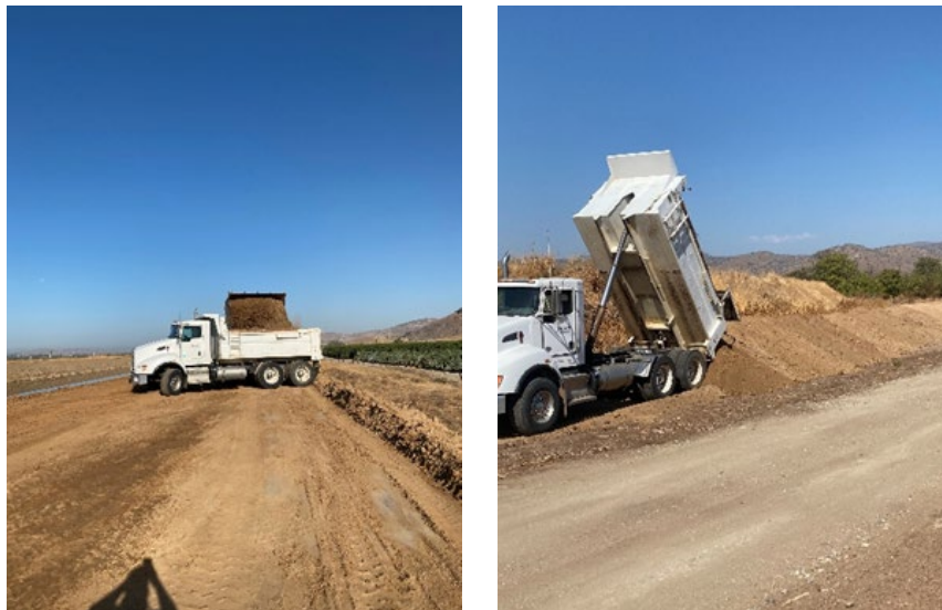
Orange Cove staff continue hauling materials off the embankment from the recent desilt project
