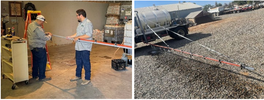
Lindsay staff completed plumbing on new boom arm for chemical applications on inside canal banks
