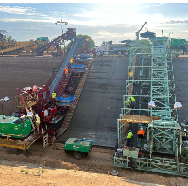
Pouring and forming of concrete lining in the new Friant-Kern canal. See more details and photos on page 3-4.
