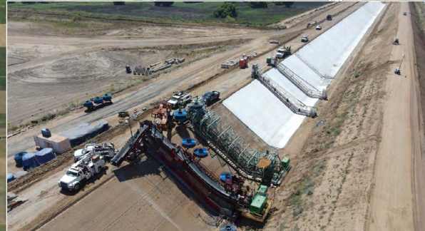
Canal lining machine north of Deer Creek on east side of new canal
