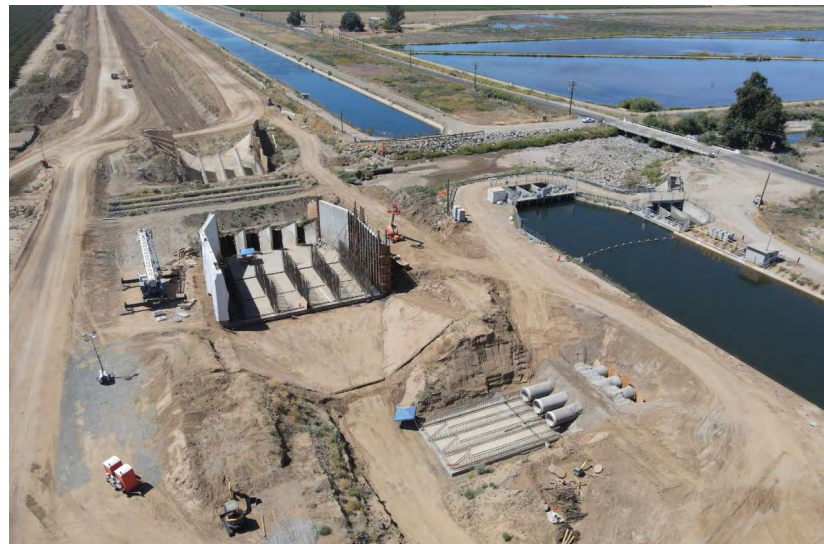
Deer Creek check structure and wasteway pipes
