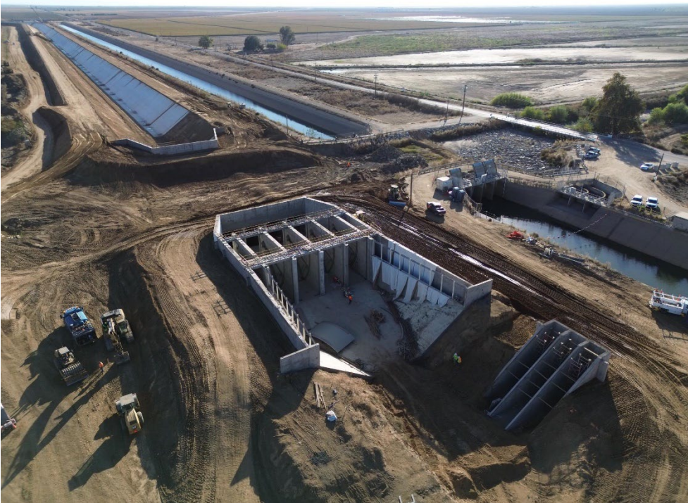
Deer Creek Check Structure radial gate arms were installed. Structural backfill conducted.
